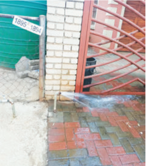
Water meter thieves are creating problems in Northam.
